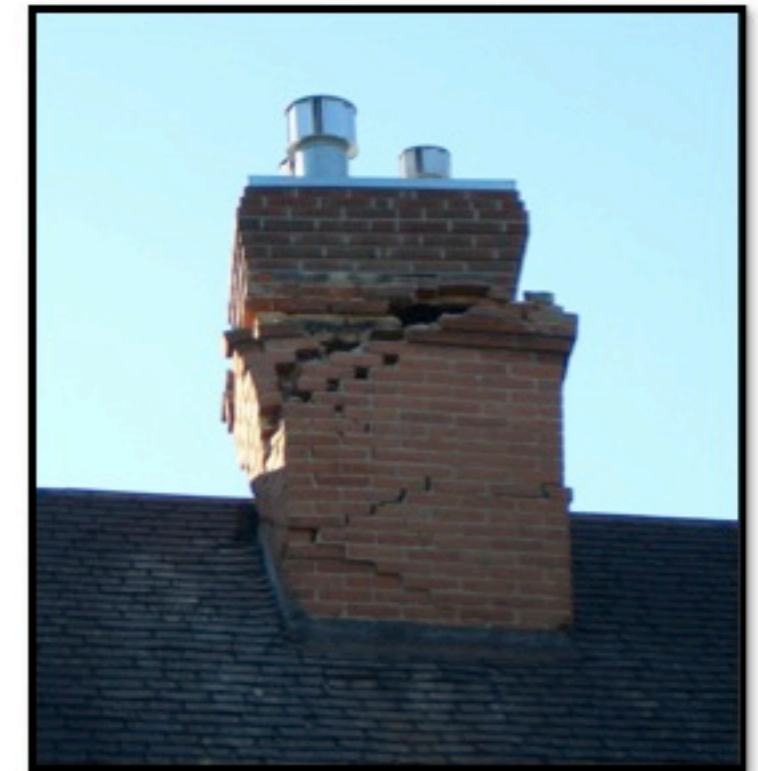
Damage from the July 25 th , 2005 quake in Dillon
